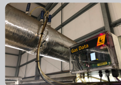
Gas Flow Monitoring
